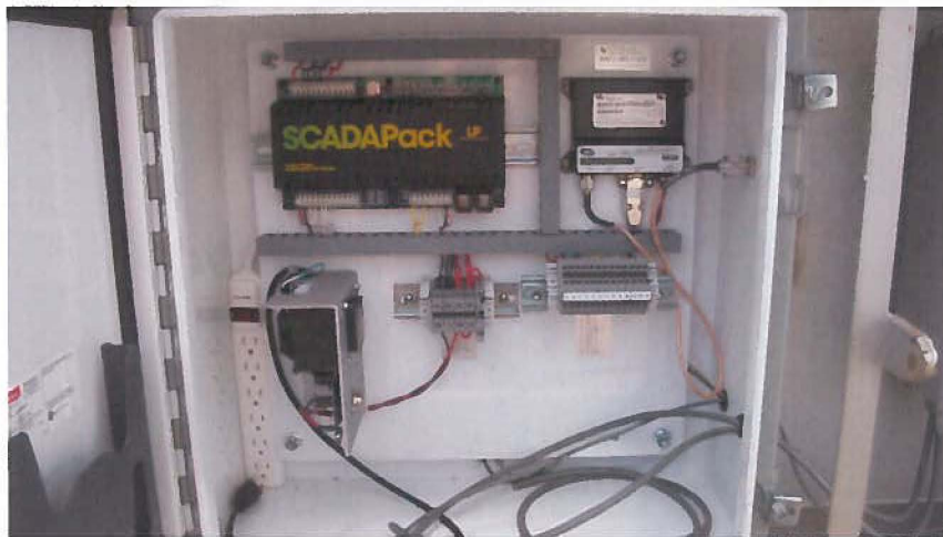
Picture 3. SCADA instrumentation.
